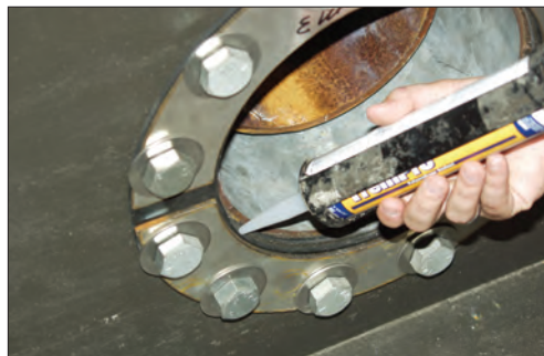
Figure 15. Caulk Exposed Galvanized Steel
