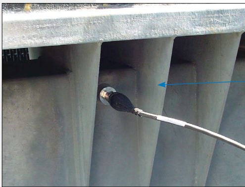
Figure 15a. Accelerometer Location - Gear Drive
