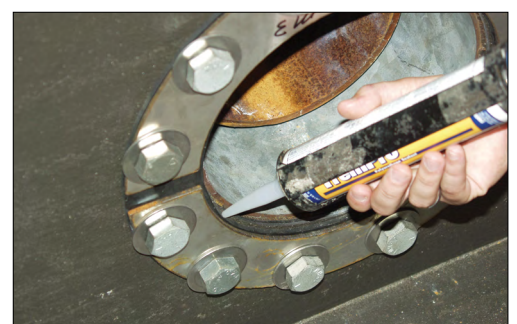
Figure 18. Caulk Exposed Galvanized Steel
