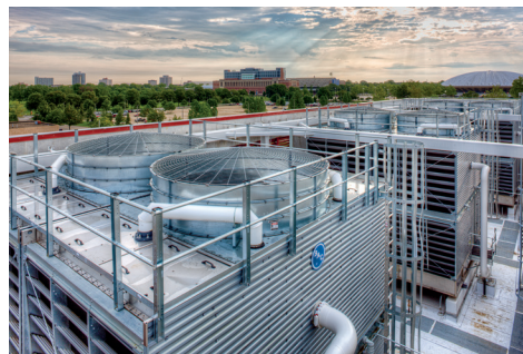
Three 31056C Cooling Towers (Photo Courtesy of NCSA)
