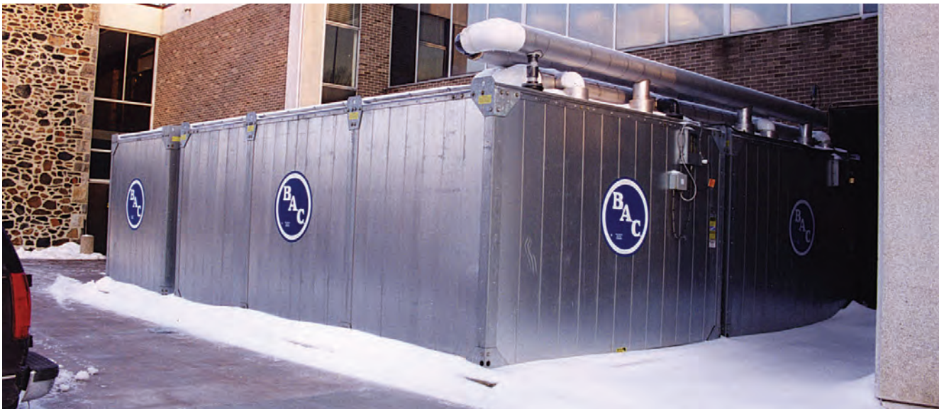
Ice Thermal Storage tanks at Catonsville Community College in Catonsville, MD, just outside Baltimore.
