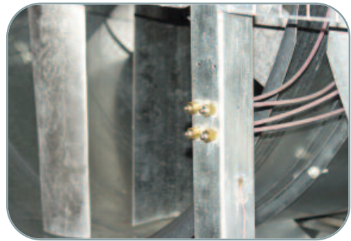
Figure 7 - Extended Lubrication Lines
