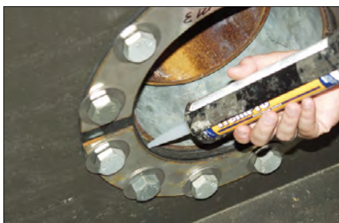
Figure 17. Caulk Exposed Galvanized Steel
