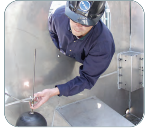
Figure 3 - Water Make-up Valve Assembly
