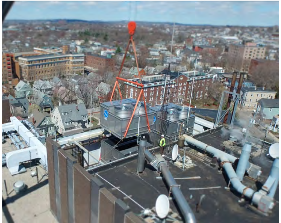
TG Gallagher stuck to a tight work schedule by replacing Cambridge Hospital's BAC Series V Cooling Towers with Series 1500 XE Models, which are designed to fit the same space with the same steel support layout but use less energy and run more quietly.
