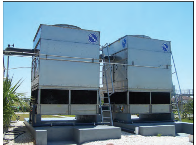
PT2 Cooling Tower
