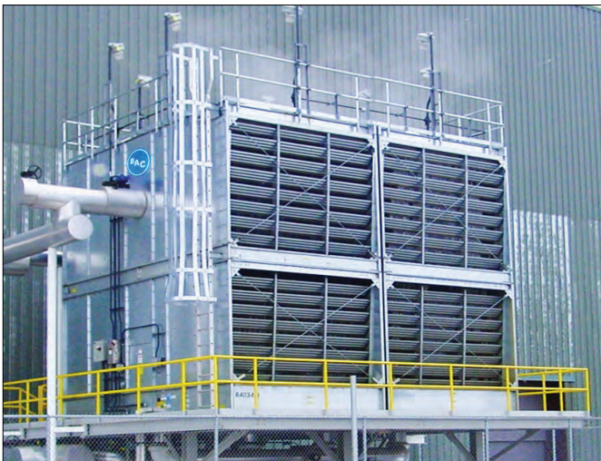
Series 3000 Cooling Tower
