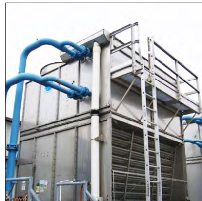
Access Platform and Ladder
