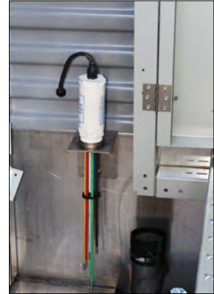
Electric Water Level Control
