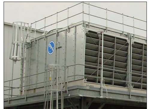
External Ladder, Safety Cage, and Handrail
