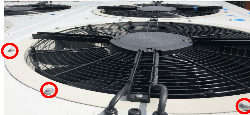
Figure 23. Fan Deck Fasteners
