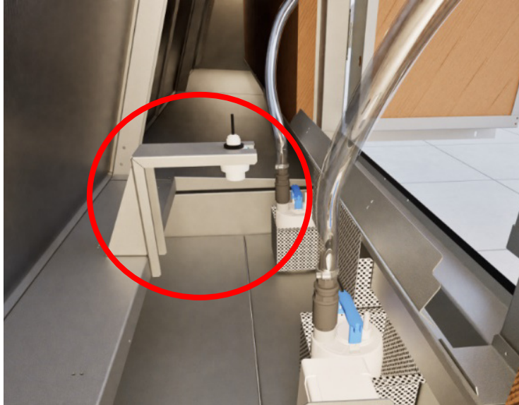
Figure 15. Sump Water Level Radar Sensor
