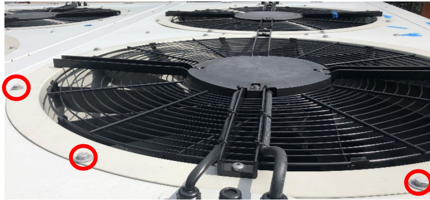
Figure 30. Fan Deck Fasteners
