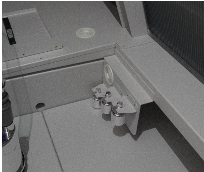
Figure 16. Sump water level float switches
